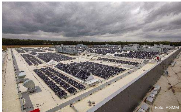
ACCUmotive Kamenz Expansion production site, Plant II,
